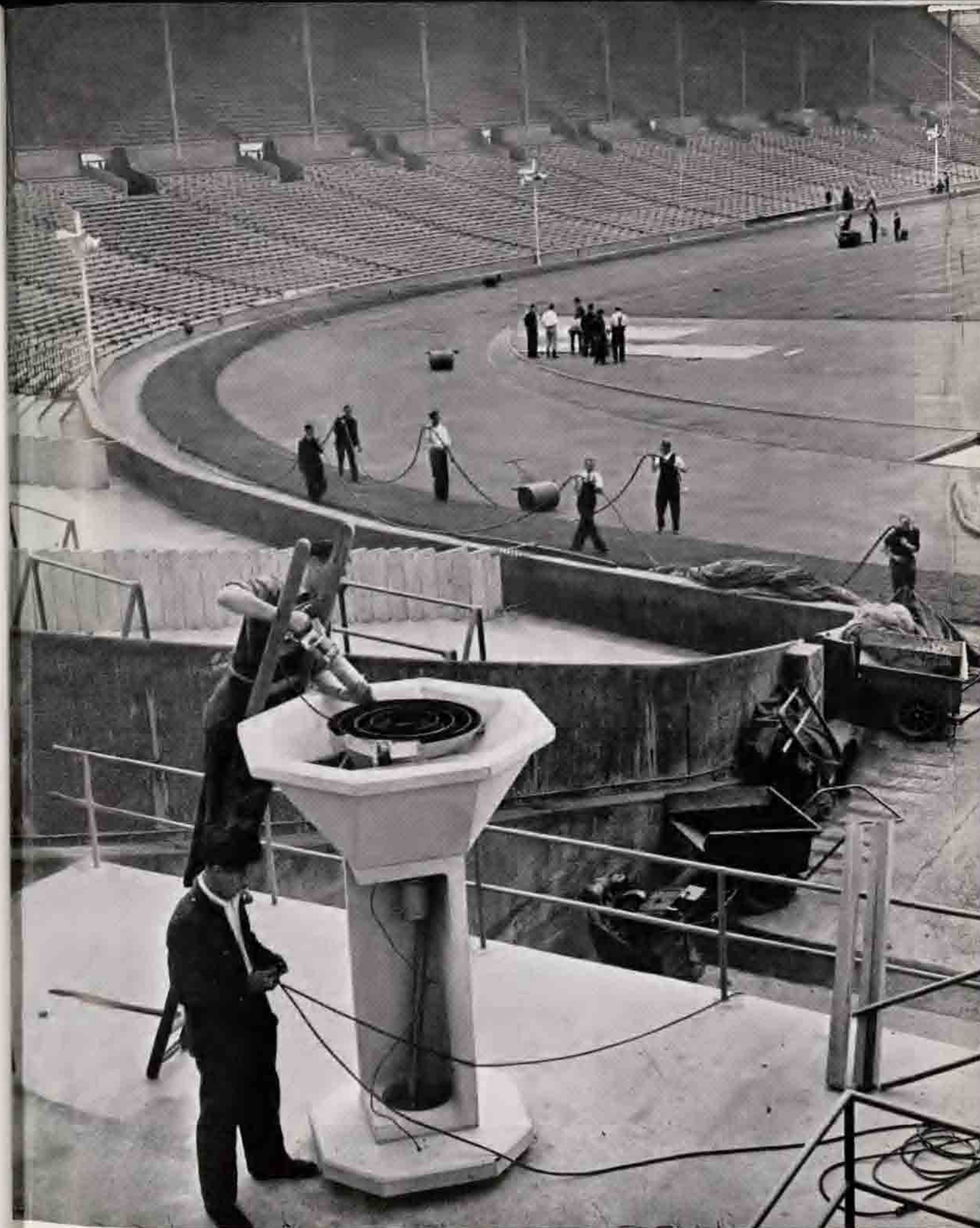
Work in progress on the preparation of the bowl for the Olympic flame at the Empire Stadium, Wembley. In the background, the finishing touches are being given to the athletic track and arena.
