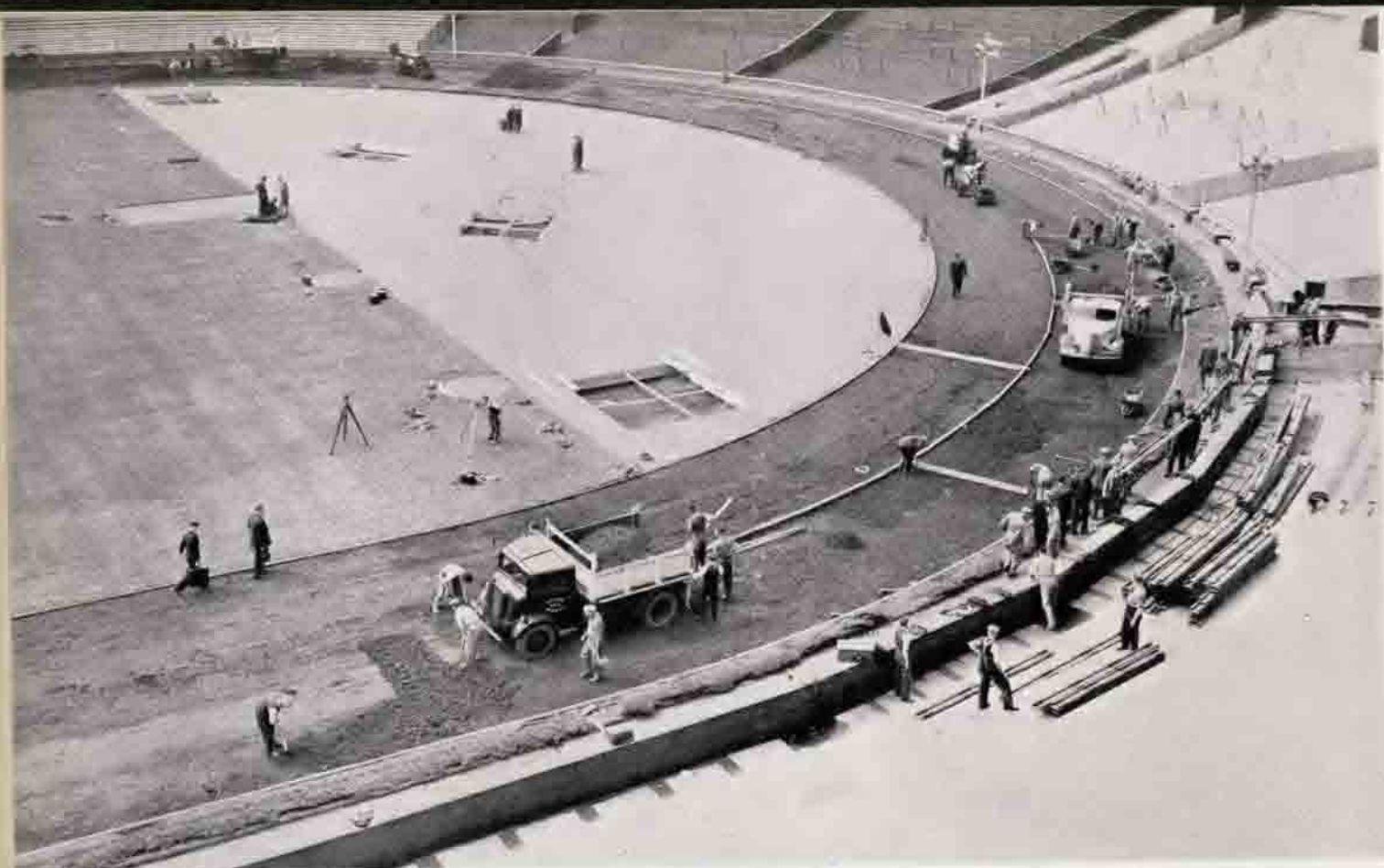
A general view of the work of laying the special track for the athletic events of the Games at the Empire Stadium, Wembley.
