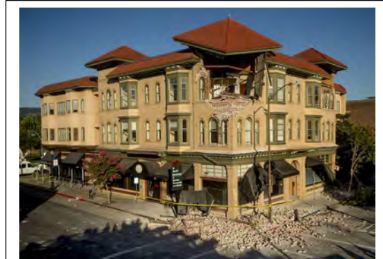
In 2014 a 6.0 magnitude earthquake occurred in the southern portion of the City of Napa on the West Napa Fault. The event was the largest earthquake in the San Francisco Bay Area since the 1989 Loma Prieta earthquake. Total damage in the southern Napa and Vallejo areas ranged from $362 million to $1 billion. Photo Credit: LA Times 2014
