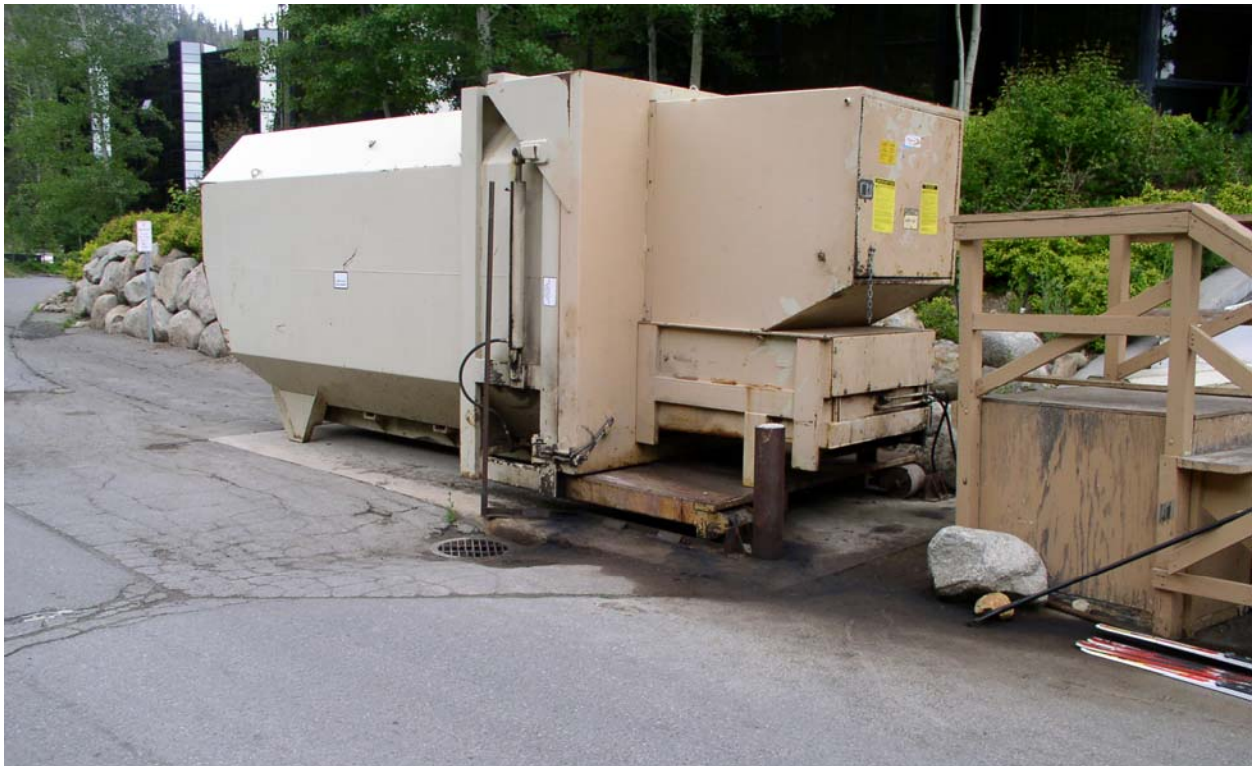
Figure 8. Leakage (“dumpster juice”) from a Compactor/Dumpster Directly into a Storm Sewer.
