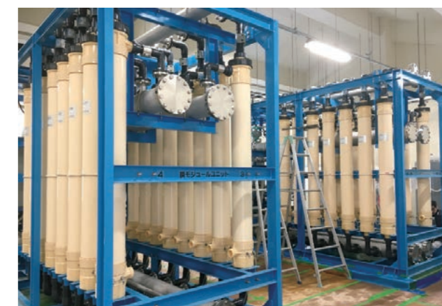
Pressurized module for wastewater treatment
