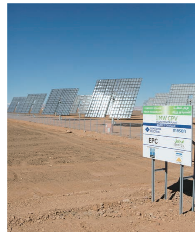
Morocco CPV project
