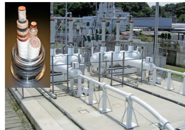
Superconducting cable project
