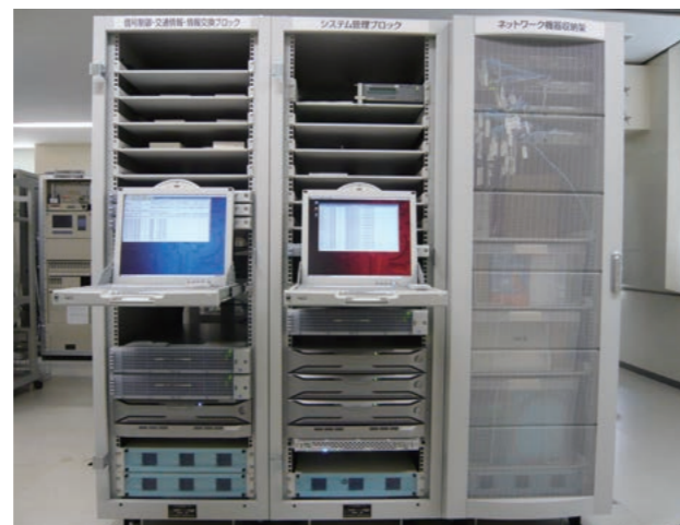
Traffic control system used by the Tottori Prefectural Police
