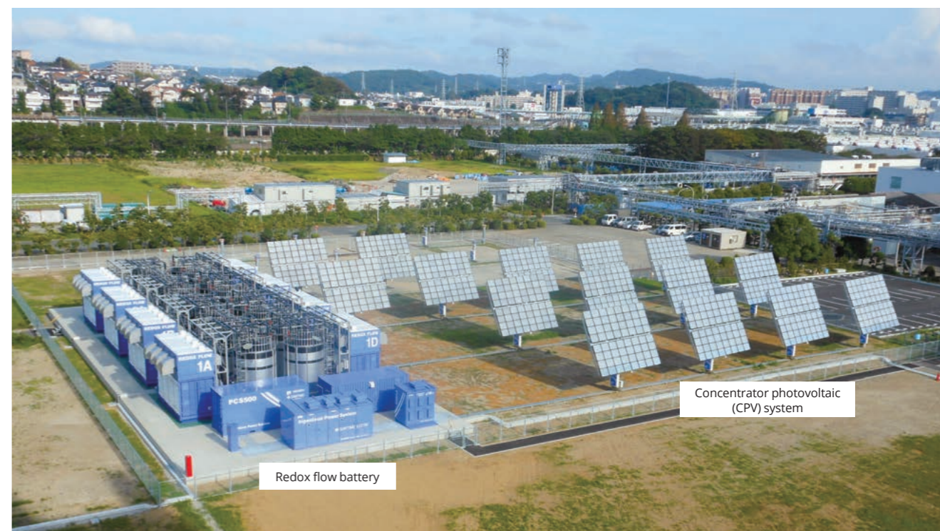
Demonstration project of a large-scale power generation/storage system (Yokohama Works)
