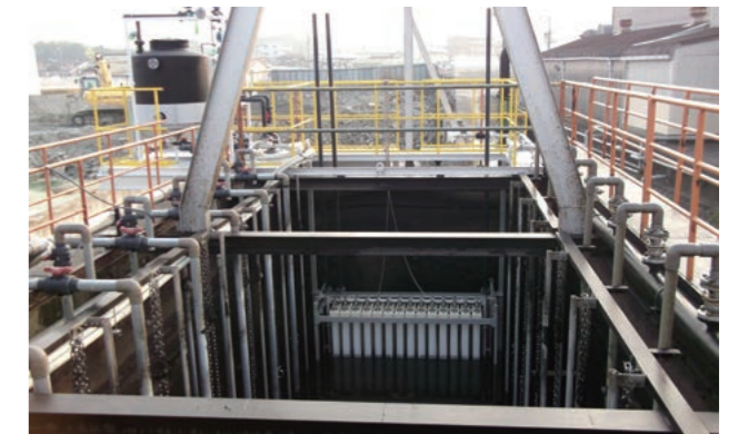
Water treatment equipment of the East Cafeteria at Osaka Works
