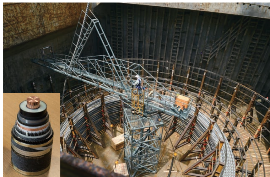
High-voltage DC transmission cable for NEMO Link Limited.
