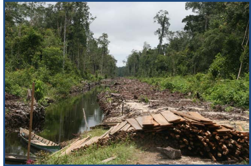
Figure 31. Photograph of recently dug canal and road from Seruyan River to PT Kharisma oil palm estate (coordinates: 2.68 degrees South, 112.204 degrees East)
