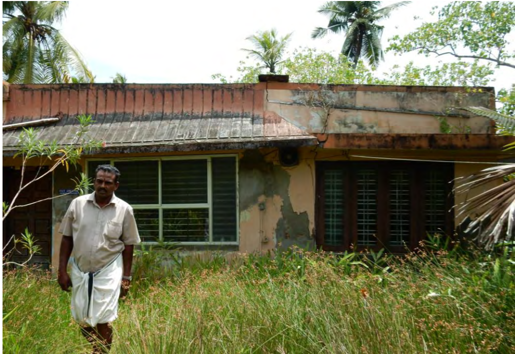
A damaged building due to land subsidence at Munroe Island
