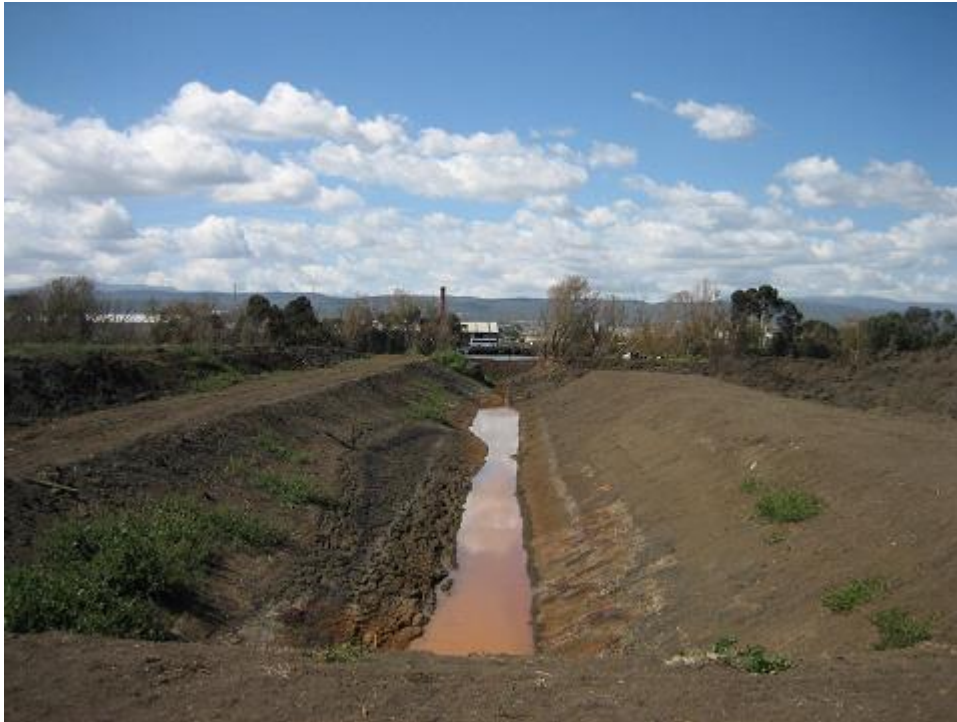
Figure 35. Photo of acid leachate in newly cut open drain between two of the silt ponds in March 2008 showing high levels of iron.
