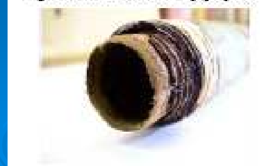
Figure 16: Corrosion of pipe joint
