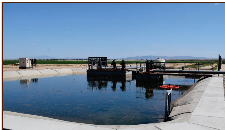
Newly-installed holding reservoir for Colorado River water storage at the east margin of AKA's California farm.
