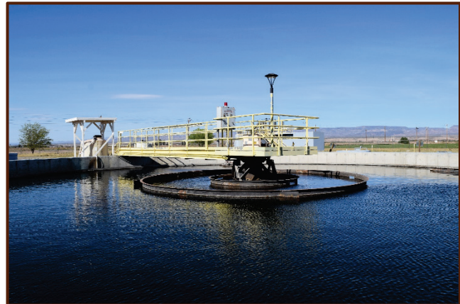
Fort Mojave Tribal Utilities Authority Municipal Wastewater Treatment Facility holding pond at the south-central Reservation; the facility serves residential, industrial, and commercial entities throughout the region of Mohave Valley and Fort Mohave.
