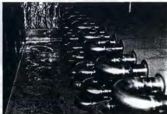
Sludge heat exchanger ▲
