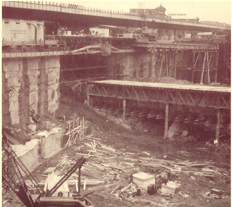
View of World Trade Center Foundation Work. H&M Tubes entering site in foreground. West Side Highway in background. Note slurry wall & tiebacks.
