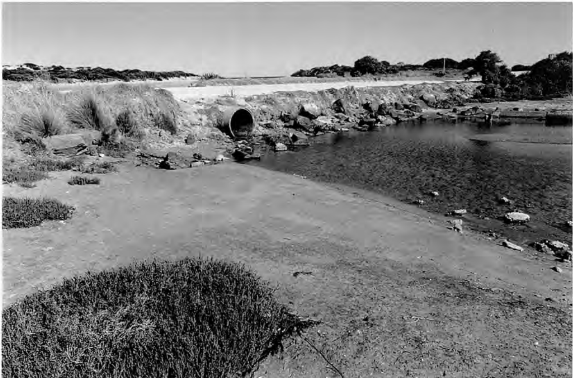
Plate 16. The small culvert on Point Impossible Road, west side of Thompson Creek, restricting tidal inundation of the Saltmarsh.
