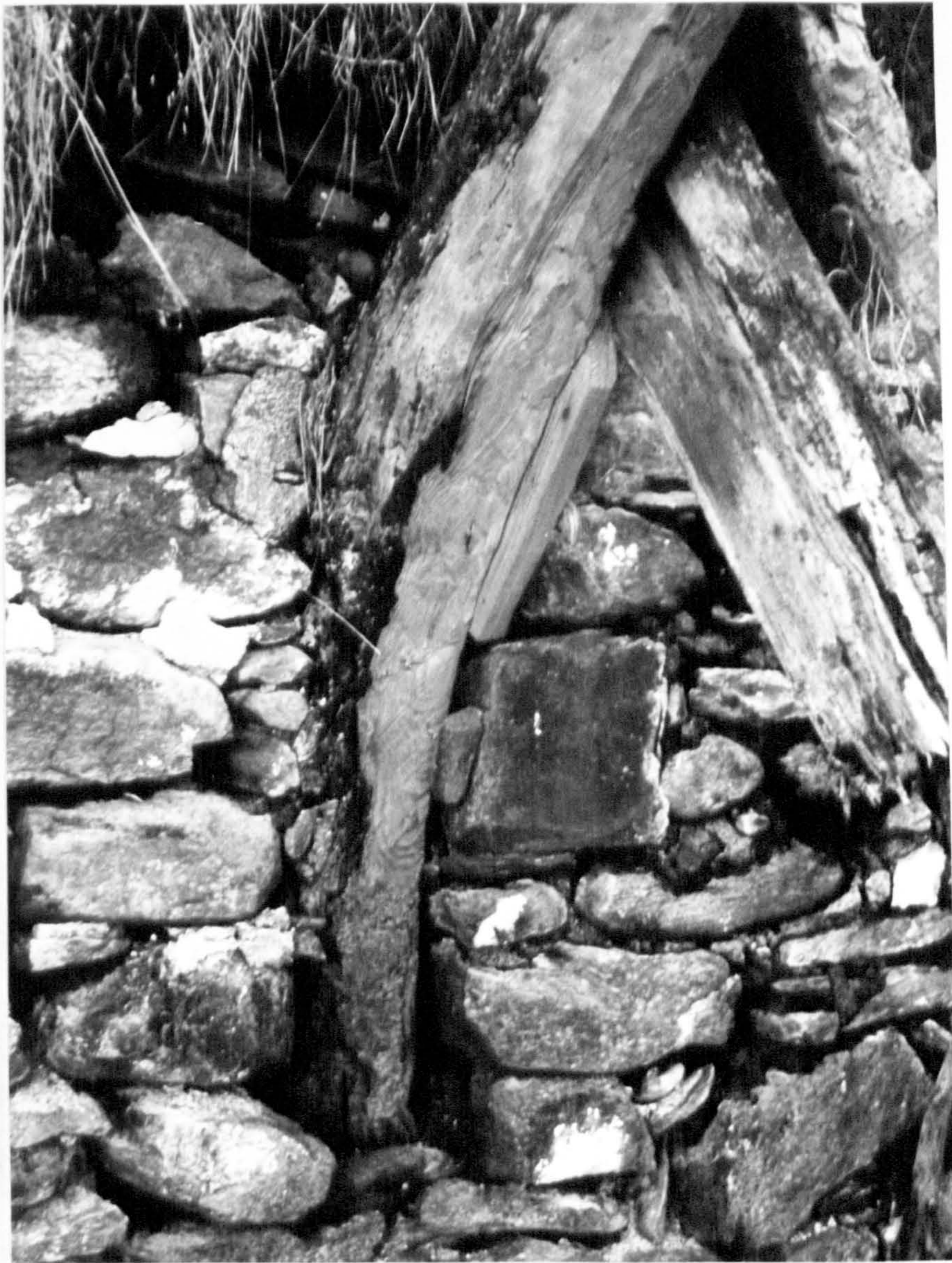
Plate 28. Foot of cruck in wall slot, central cruck, south wall of Section A 1 , Building A in Cluster B on Cuiltrannich, 1966.
