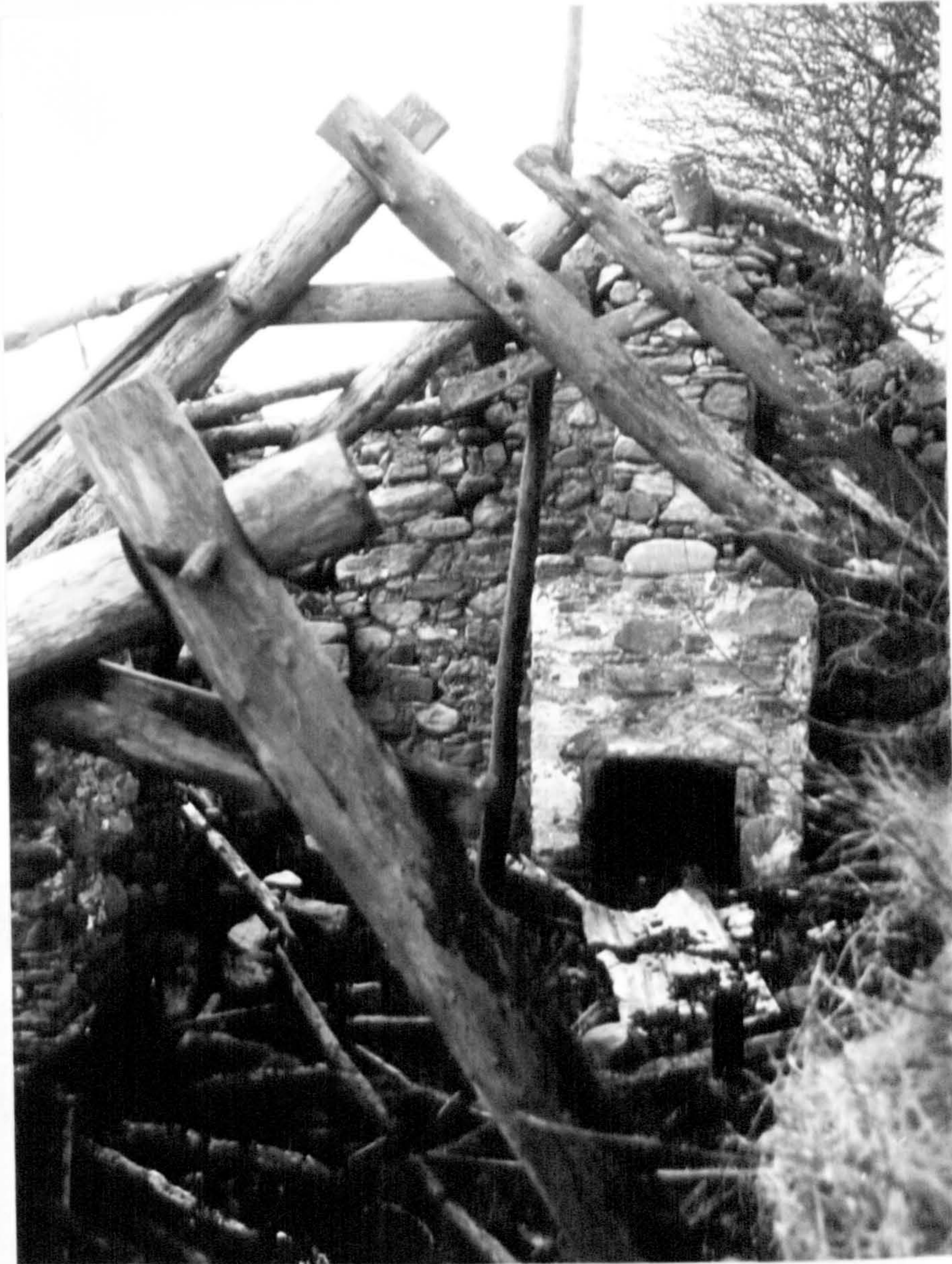
Plate 26. Interior of Building A in Cluster B on Cuiltrannich in 1966, looking west. The outer, rounded side of the cruck couples can be seen from this direction. This section of the original byre-dwelling had a hearth located just off the photograph in the foreground, with smoke going out through a probable 'hanging lum', the outer aperture of which can be seen in Plate 20. The gable-end fireplace is a secondary structure, 'added on' to the wall face with a chimney and chimney pot still visible. A fallen ridge-pole or purlin is standing upright in front of the fireplace.
