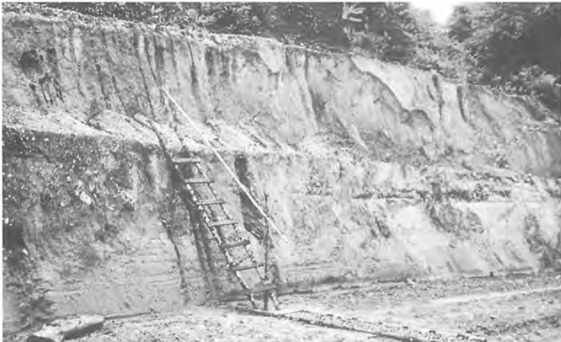
Figure 5. Within months after being exposed and contoured, many road cuts began to erode. Since the remaining subsoil lacks fertility, vegetation has been unable to recolonize. Photo: Scott Poynton, 8 March 1998.
