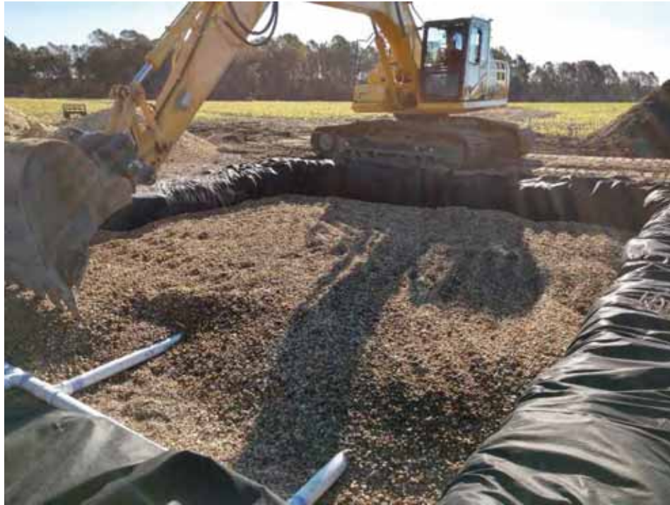
Figure 7: Blind inlet example showing the filter (gravel) being placed over the subsurface perforated drainage pipes.
