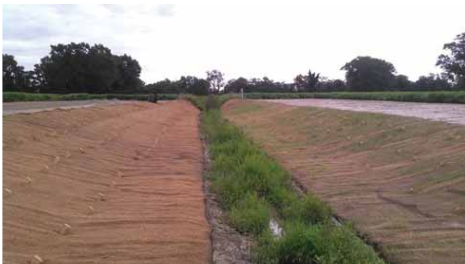
Figure 16: Two-Stage Ditch example showing the extended benches within the ditch. This two-stage ditch is located in Talbot County, MD.
