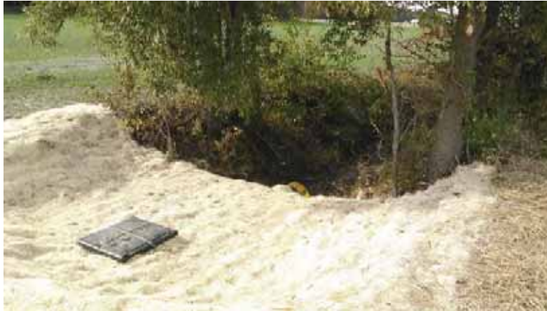
Figure 15. Structure for water control installed in a ditch to help control water level and increase nutrient removal within the ditch.
