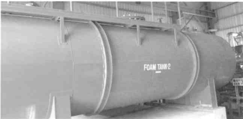
Fig. Fire station & Fire tender
