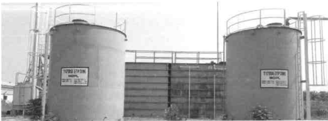
Fig. Effluent Treatment Plant (50 KLD)
