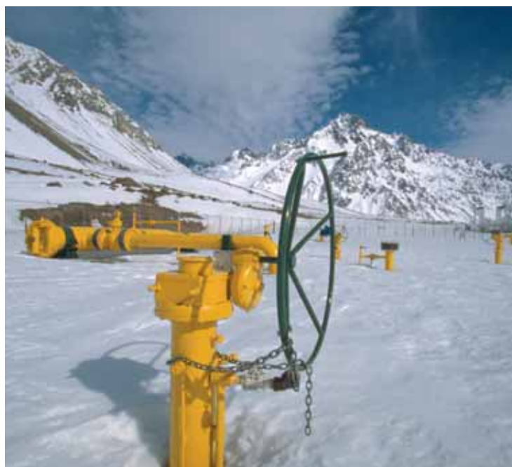
Chile: this 460-kilometer gas pipeline runs from Argentina's gas grid across the Andes divide to the Chilean capital, Santiago.
