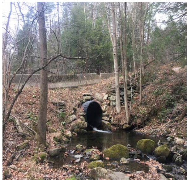
Chester stakeholders had many concerns regarding the impact of flooding on infrastructure such as bridges, roadways, and culverts.
