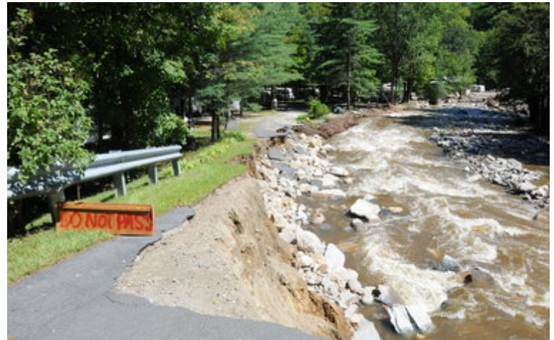
Walker Brook flooded during Hurricane Irene and caused extensive damage to the Walker Island Campgrounds.
