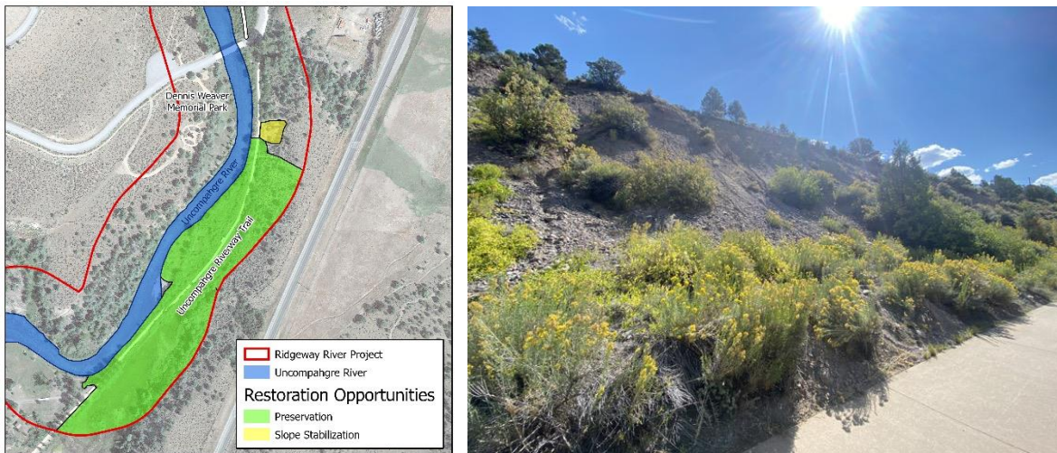
Figure 17 - Potential slope stabilization location east of Dennis Weaver Park (left). Steep slope with active erosion occurring. Revegetation recommended to stabilize slope.
