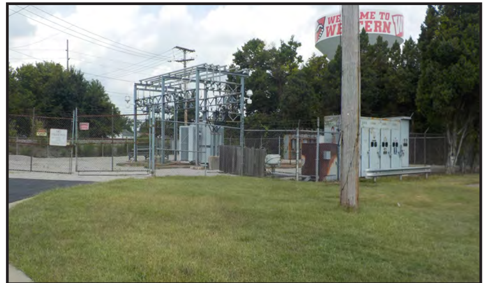
Photo 12: Electrical substation, field identified potential hazardous materials site, University Boulevard; facing north.
