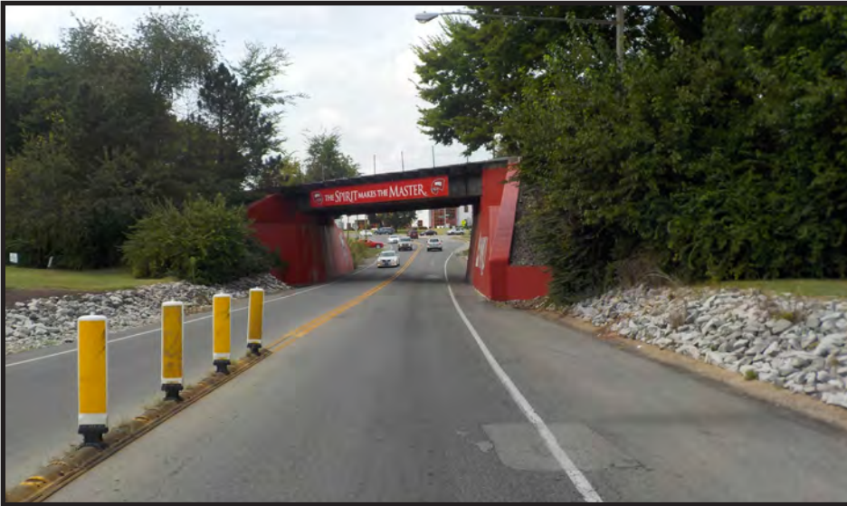
Photo 21: CSX railroad bridge over US 68X / US 231X in study area; facing west.
