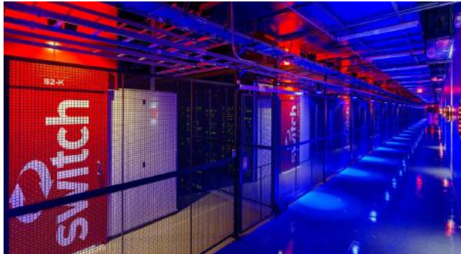
Switch, Inc., IFM
