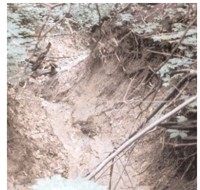
Figure 47. Photograph of downcutting just downstream from pipe shown above.
