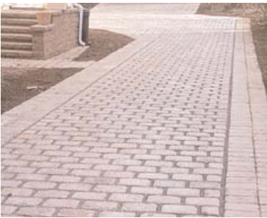
Figure 39. Photograph showing permeable paving system for residential driveway (Elmhurst, IL).
