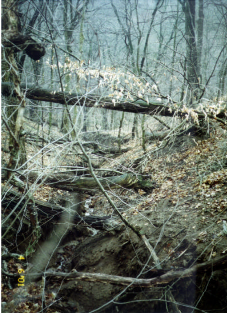
Photo 3 Study Area #12 - Sleepy Hollow Road - Looking DS from end section. Erosion cut is about 8-ft deep and 8-ft wide (triangular section) (0_pic21.jpg)
