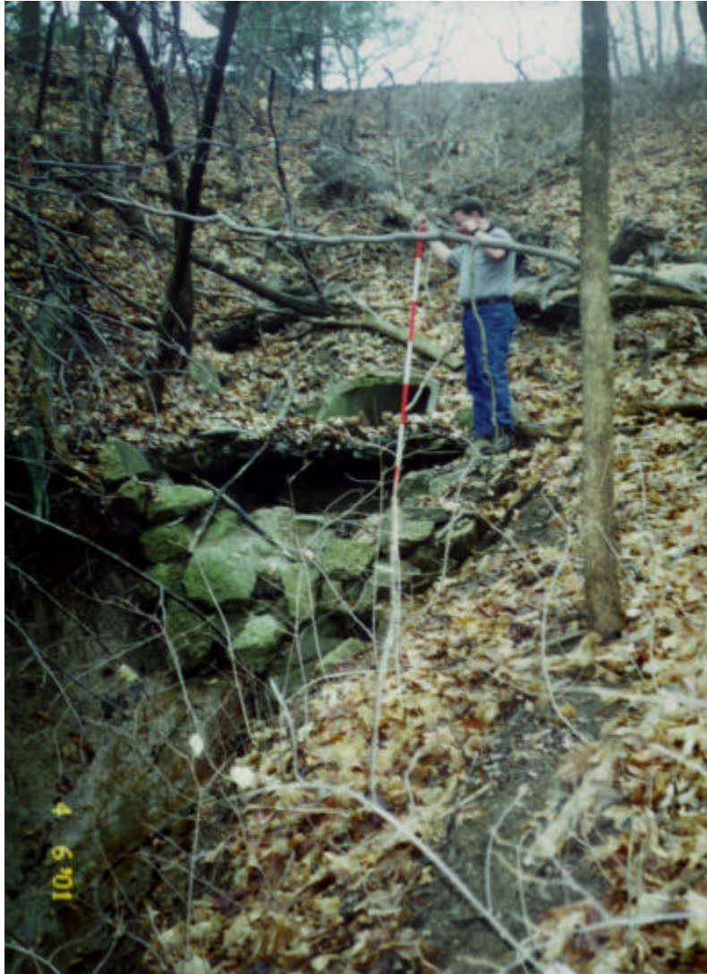
Photo 1 Study Area #15 - Grand Oak Drive - Erosion DS of end section and riprap is about 8-ft deep. (0_pic12.jpg)
