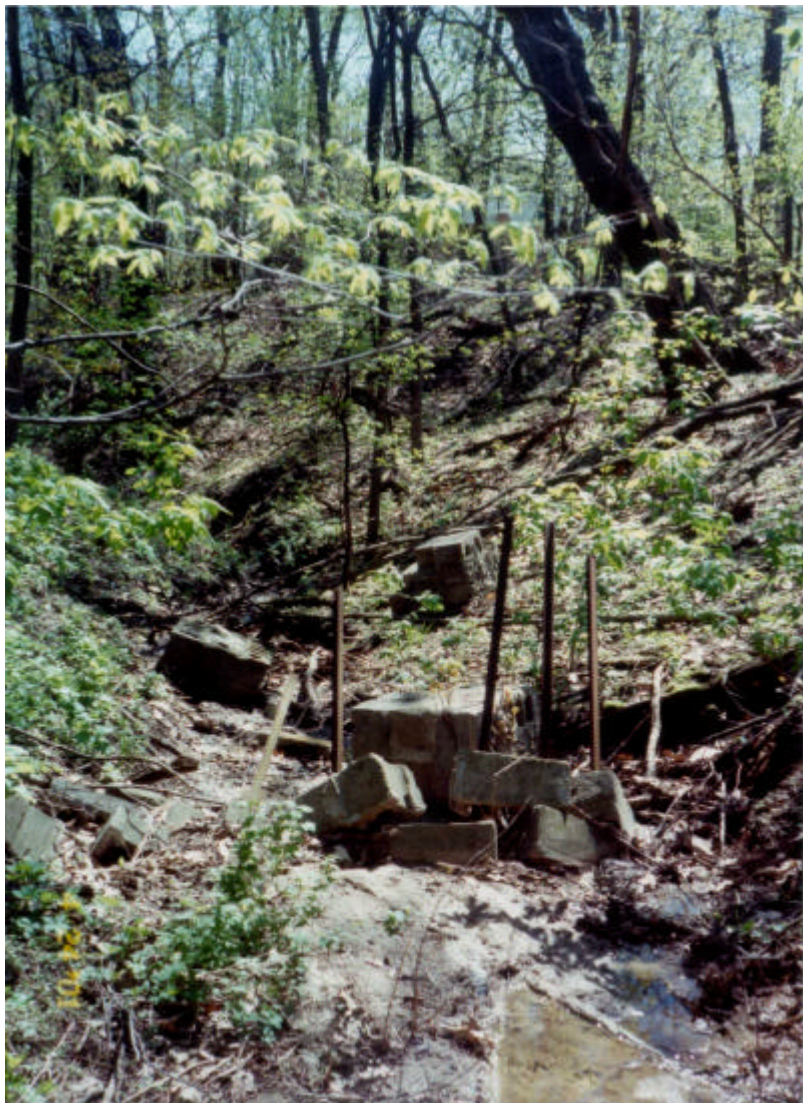
Photo 8 Study Area #8 - Knoxville Avenue - Failed grade control structure (concrete block and fence posts) further US of confluence. (2_pic24.jpg)
