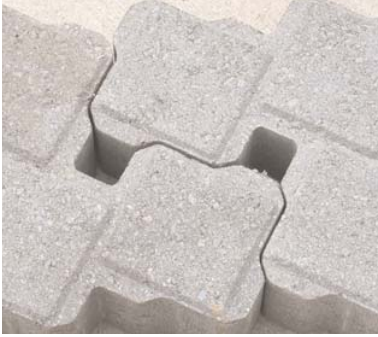
Figure 38 (above). Interlocking porous pavement infiltrates water through small square openings (installed at Dominican University, River Forest, IL).
