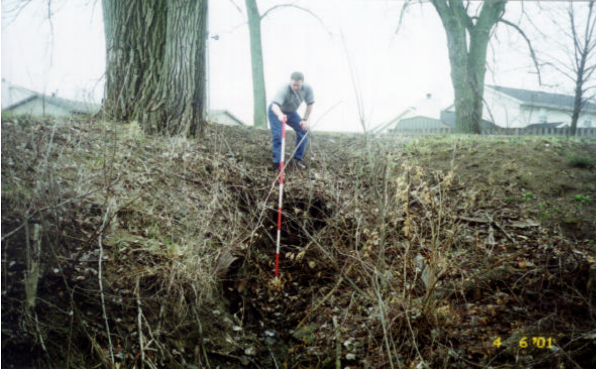
Photo 5 Study Area #4 - Ravinswood Dr/Ravin Rd - Looking US at head of ravine. One 18" diameter and one 36" diameter CMP outlet at this point. (0_pic07.jpg)
