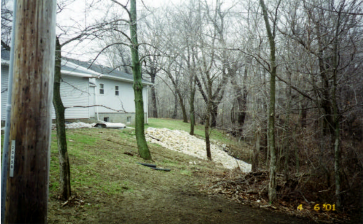
Photo 6 Study Area #4 - Ravinswood Dr/Ravin Rd - Looking DS from head of ravine. Deep cuts below culvert (0_pic06.jpg)
