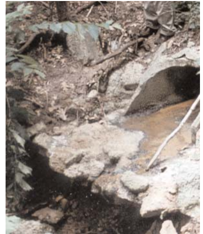
Figure 46 (above). Photograph shows downcutting at the discharge point of concrete pipe.
