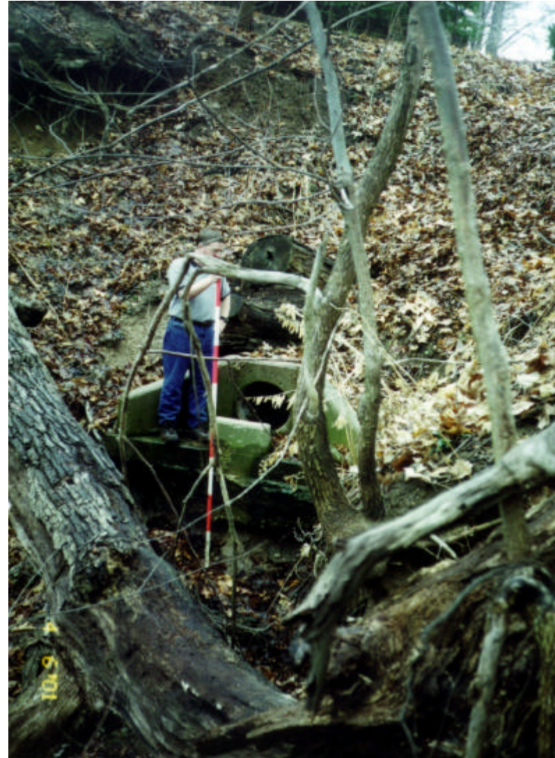
Photo 2 Study Area #12 - Sleepy Hollow Road - SS outlet: 18" RCP and CIP end section with disipation block. Slope is undercutting end section 4-ft deep. (0_19pic.jpg)
