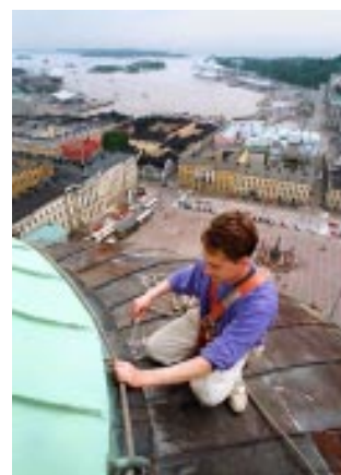
Helsinki Cathedral under renovation. Outokumpu has developed the Nordic Green™ method for artificial patination of copper roofing on site. Shiny copper sheets acquire a classic green patina in days.
