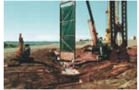
The 3.1 km long underground insulation wall being built around the Kokkola zinc plant waste area is due for completion in 2000.
