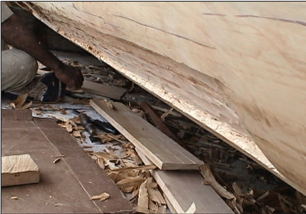
Figure 141. View of a large soft area to be replaced. New boards for use in the replacement were visible on the ground.
