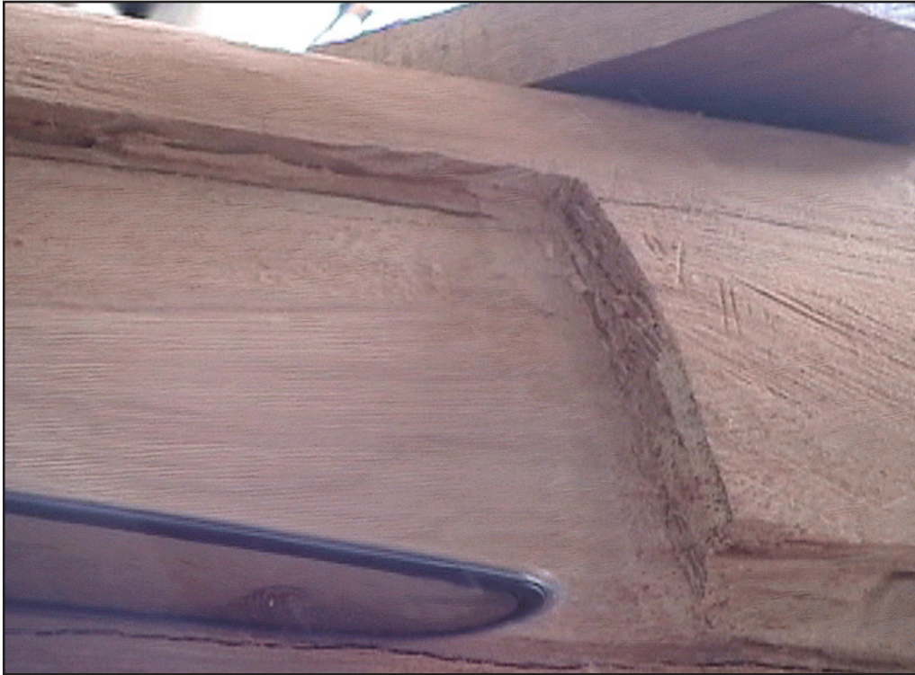
Figure 140. At least an inch in depth was removed from one of the endcovers by grinding it away with a chainsaw.
