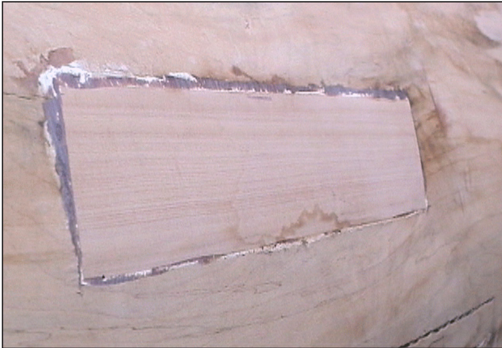
Figure 138. After the rotten wood was removed, good wood was glued in its place with epoxy.
