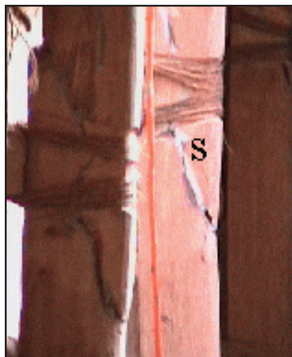
Figure 86. Note the angled scarfing (s) of the upper rib piece to the lower rib piece. Lashings were placed over these joints, here to join the ribs to the comb cleats behind.
