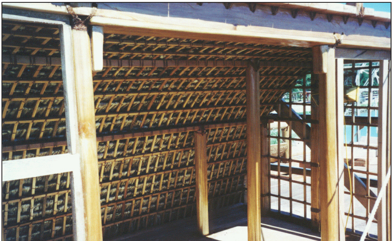
Figure 147. The almost completed fale was outfitted with pandanus thatching on the back.
