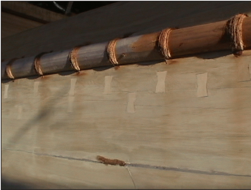
Figure 142. Butterfly plugs were used to prevent further split or checking.
