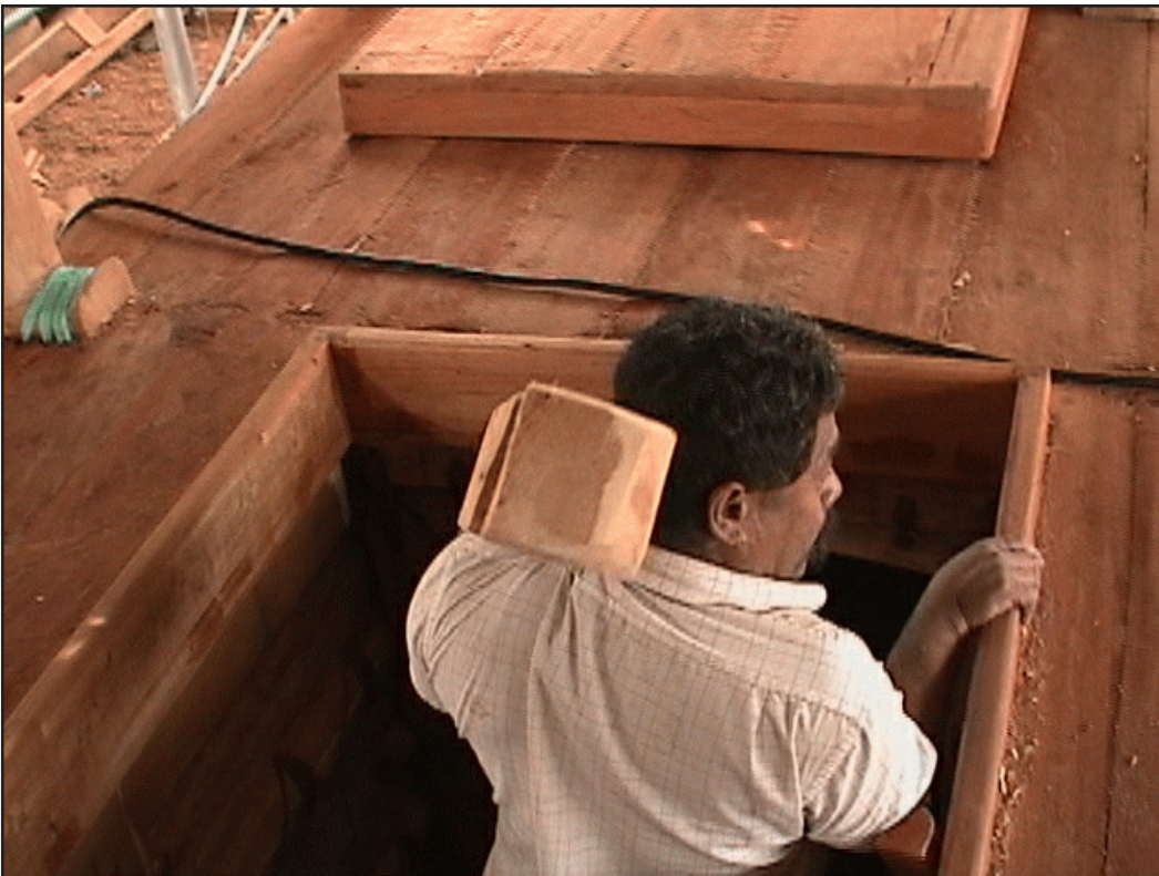
Figure 107. This worker entered a hatch carrying a rib for fitting and installation. Note the hatch cover just in view at the top.
