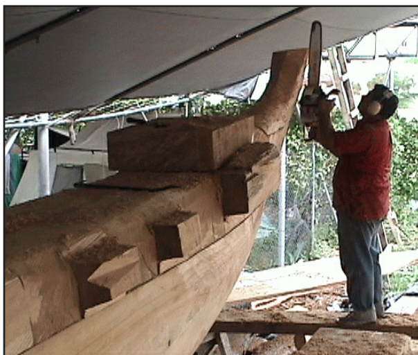
Figure 92. These roughed-in runners on katea prow deteriorated.
