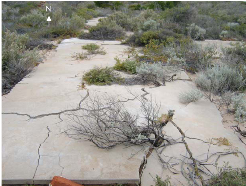
Figure 9.26. ‘T’ shaped concrete pad of the administration building (F2). Photograph taken looking north.
