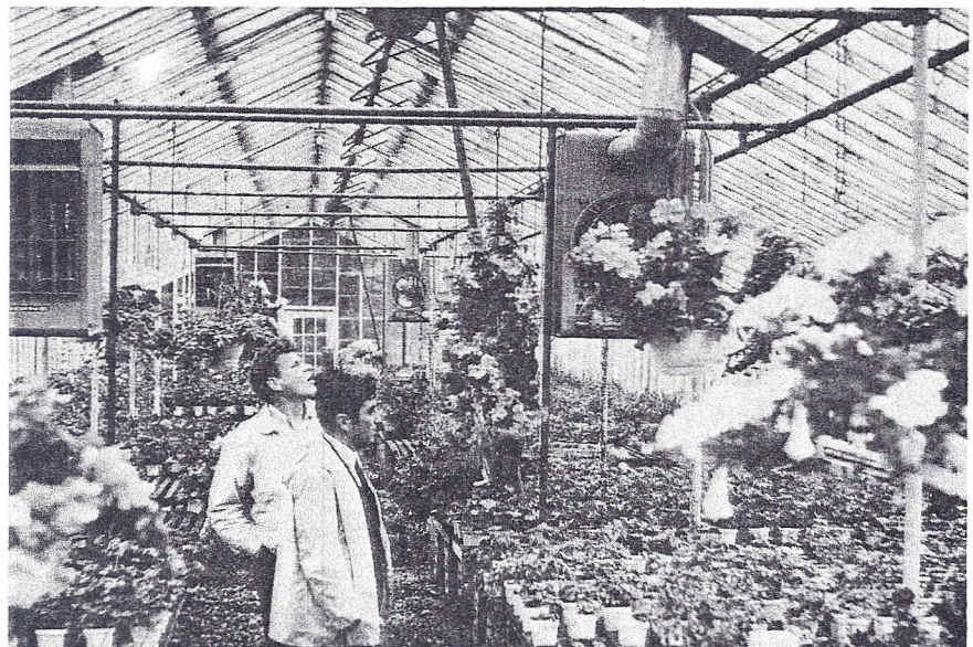
Fig. 14. Unit heaters can provide HAF. The fans are not efficient since the air must move through the heater and turbulence decreases air speed. Also note that two heaters (near left and far right) are too close to the end walls. They should have been mounted at the mid point of the house.
