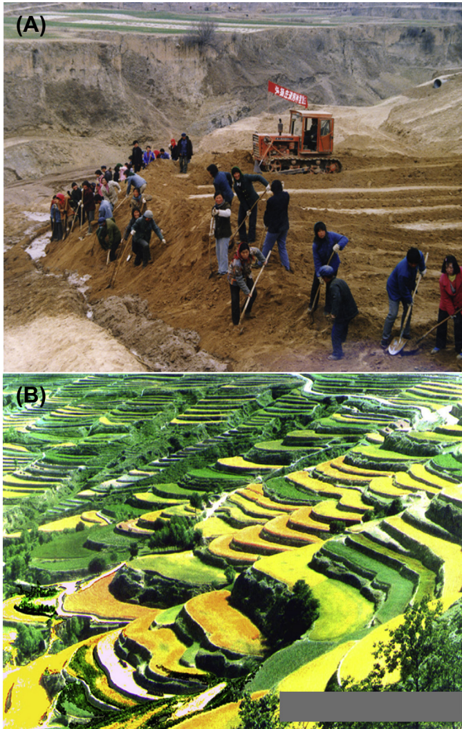
Figure 2.8 (A) Land leveling, and (B) contour terraces in northwestern China. Photos provided by Soil and Water Conservation Department, Ministry of Water Resources, China. (For color version of this figure, the reader is referred to the online version of this book.)
