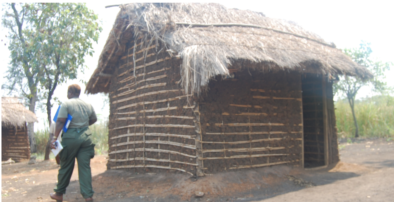
Figure 26: Picture showing one of the dilapidated staff structure which was later upgraded
