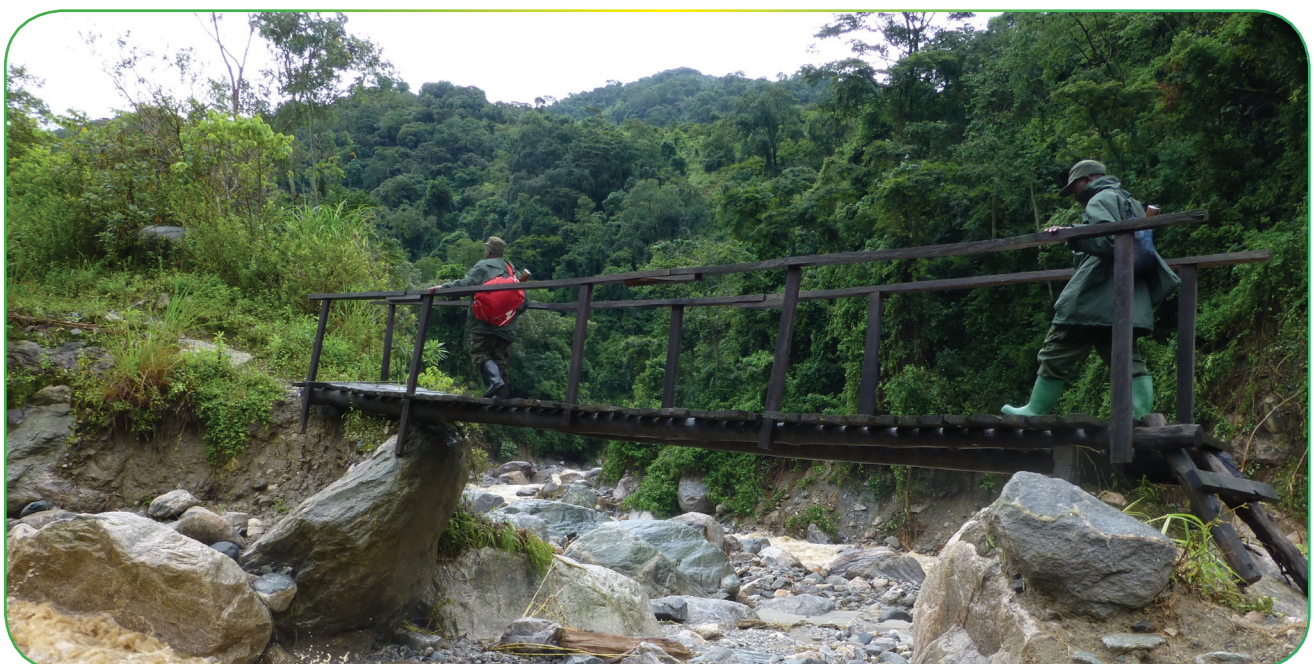
Plate 11: Photograph showing a washed out bridge due to floods
