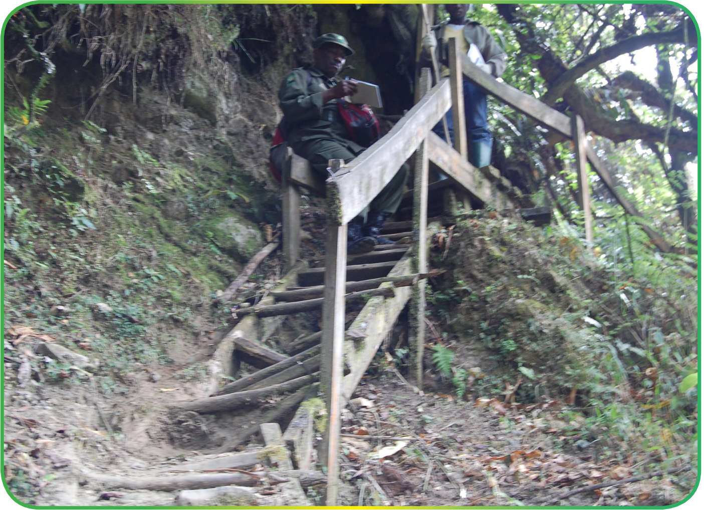
Plate 22: Photograph showing dilapidated ladders along a tourism trail
