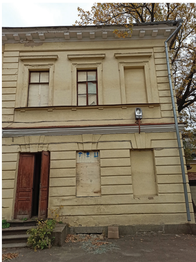
Fig. 5. Broken backyard windows temporarily boarded with plywood and cardboard
