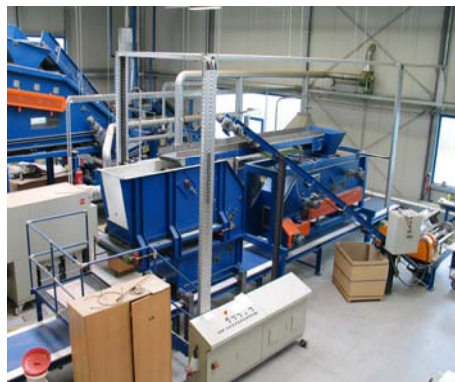
Figure 3: Pilot plant station for three layered particleboards
