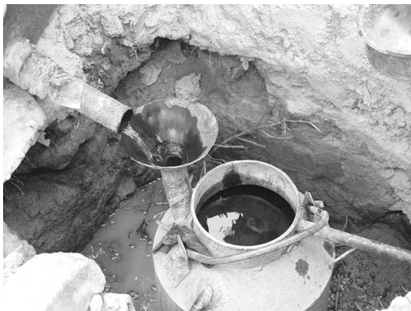
FIGURE 6.8 The converted milk can receiver (oil separator) used in India.
