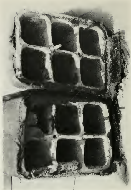
FIG. 8. SAME JOINT SHOWN IN FIG. 7 BROKEN OPEN AND SHOWING OBSTRUCTIONS IN DUCT.
