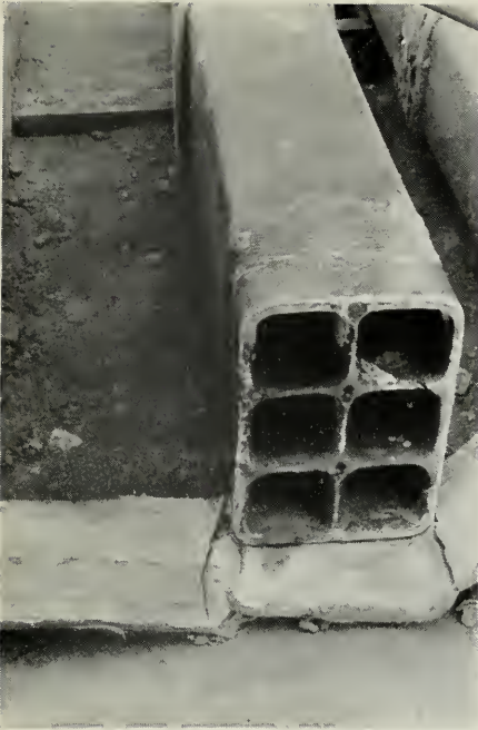
FIG. 9. MORTAR BANDAGE JOINT BROKEN OPEN. INTIMATE CONTACT INDICATED BY SCARIFICATION OF CONDUIT MARKED ON THE BANDAGE.
