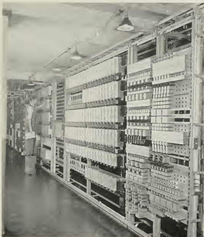
FIGURE 6. SELECTOR FRAME AND RELAY EQUIPMENT FOR MISCELLANEOUS CIRCUITS.
