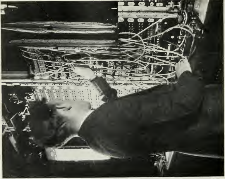
A TEST-BOARD EXPERT KEEPS WATCH FOR TELEPHONE CIRCUIT TROUBLES.
