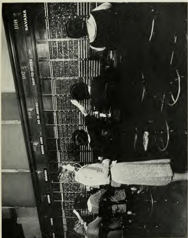
THE TRANSOCEANIC SWITCHBOARD WHERE TELEPHONE CONNECTIONS ARE MADE WITH OVERSEAS COUNTRIES AND SHIPS AT SEA.
