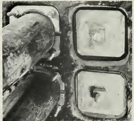
FIG. 12. DUCT PLUGS INSTALLED IN CENTRAL OFFICE VAULT.
