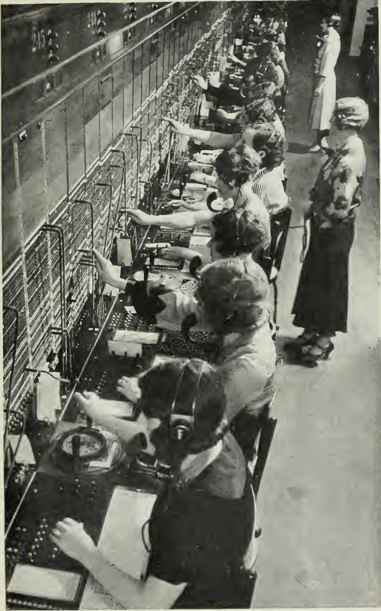
A LONG-DISTANCE SWITCHBOARD.
