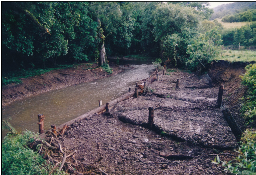
Photo 6. Bend re-alignment structure, Myall River, Mid-North coast of NSW, late 1990s. The development of a break-out point has been prevented by re-aligning the main channel using a hardwood log front wall, backfilled with point bar gravel & chainmesh laterals. The chainmesh catches flood debris & encourages deposition on the created bench, which in turn leads to the natural regeneration of native riparian plants.
