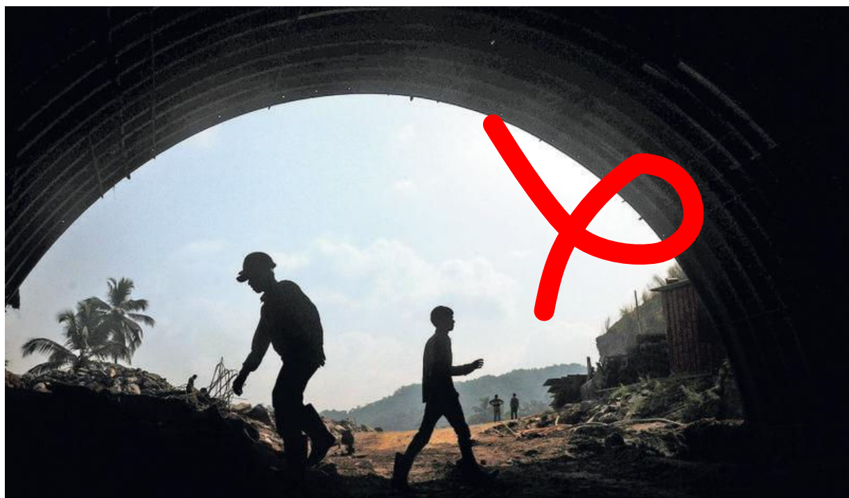
Work in progress: Workers constructing one of the two tunnels in the Kuthiran hills in Thrissur district of Kerala on the Salem-Kochi National Highway 544. The 965-metre structure is part of the six-laning of the stretch. ■K. K. MUSTAFAH
