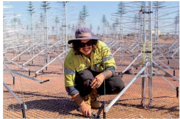
Figure 9b. Installing antennas of the Aperture Array Verification System, a testbed for SKA-Low, at the MWA site (credit: ICRAR/Curtin University).
