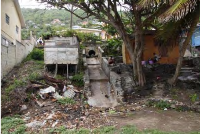
A drainage canal on Bequia Island dumps trash and sediment 50 m inland from the shoreline. Photo credit: Mike Seager
