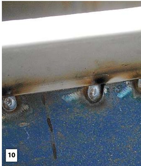
10 The window frame was clamped into the barrel and the two were plug welded together with the MIG welder; if no welder is available, pop rivets would do the same job.
