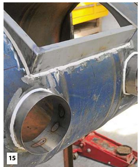
15 Once all the welding had been done, all the new seams were caulked around to seal them to avoid dust in the workshop and allowed to dry.
