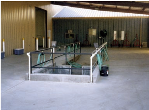
The redesigned and greatly improved wash pad at Prairie Dunes Country Club provides adequate collection and filtering of wash water. Identifying problems, choosing the most environmentally responsible treatment, and implementing a solution are a key focus area for Audubon Cooperative Sanctuary Program for Golf Course members.
