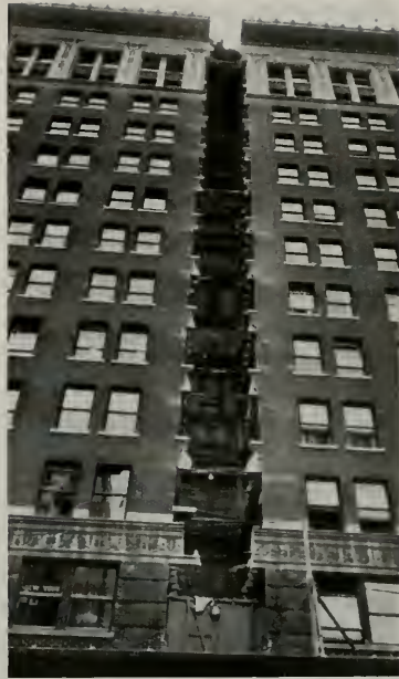
Commercial Exchange Building, Los Angeles, as it appeared after an 8½ ft. slice had been cut out of the structure.
