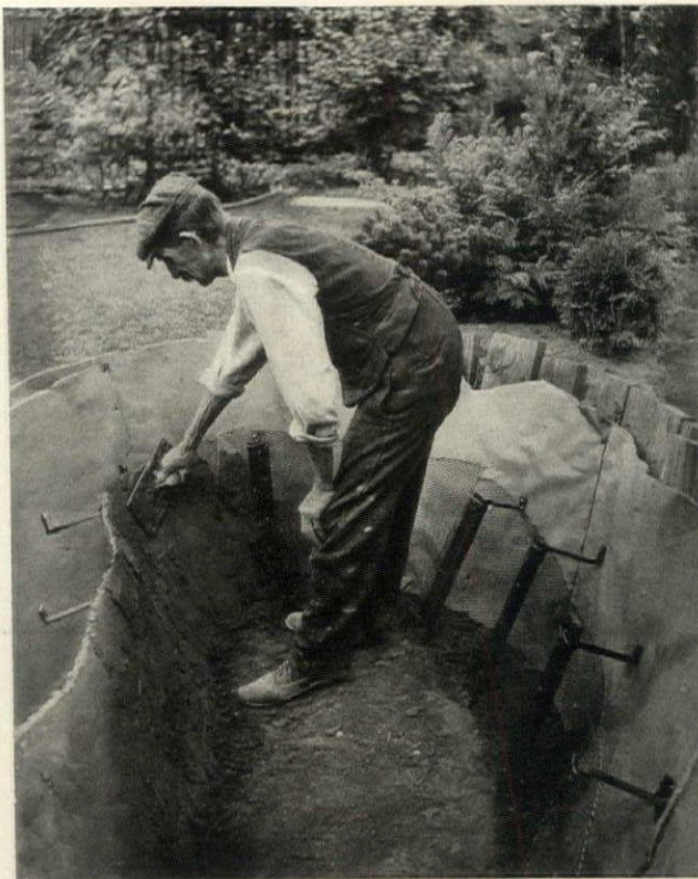
The site of the pool should be excavated to a depth of 2' or 3'. Concrete makes a good lining if a fairly rich mixture is used
