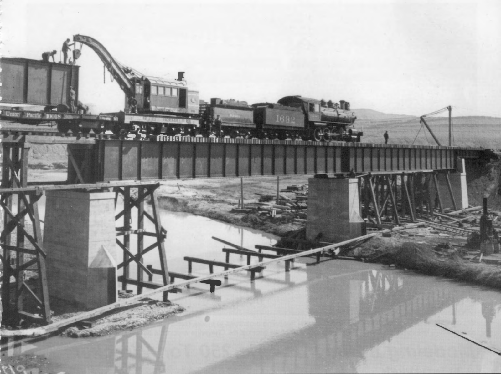
New wrecking derrick 02801 and its associated coal tender are helping construct the bridge across the North Platte River at Fort Steele, Wyo., in 1901. The 40 ton derrick car was built by Industrial Works in 1901 and renumbered to 03054 in 1919. The 24' 2" long car weighed 133,000 pounds, and had a steel underframe and a wood superstructure. Using wrecking derricks to help do work such as place girders on bridges was a logical use for equipment such as this, which was, hopefully, not being used very frequently to clear up wrecks. Note how the bridge is being constructed, with a temporary wooden falsework used to build the bridge being replaced by the permanent steel girders. Stimson photo Wyoming State Historical Society
