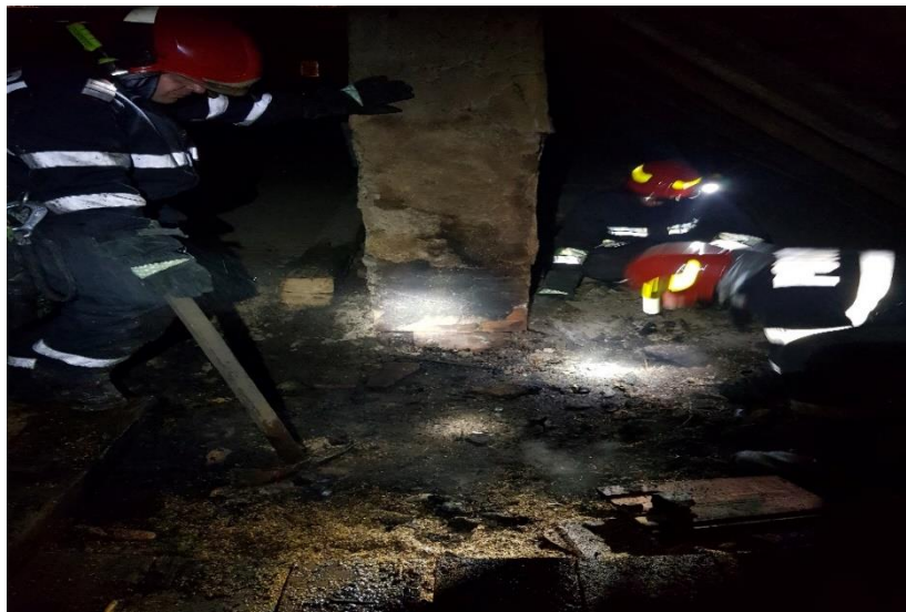
Ignition of a beam in the bridge of a house Recaş because of a chimney
