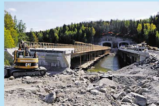
The concrete for the northern bridge at Sepänniemisalmi has been cast, and the southern bridge is open to worksite traffic. Photo: E18 Muurla - Lohja Motorway/Jouni Saaristo
