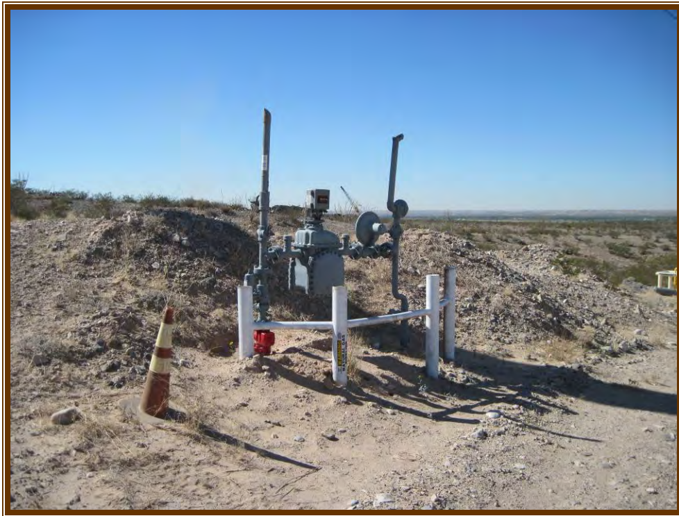
Photo 5. View gas pipeline on Border Steel Road.
