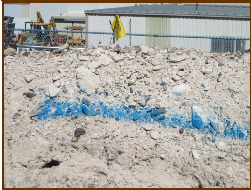
Photo 6. View of marked gas pipeline along Border Steel Road.
