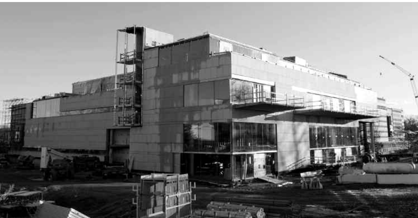
Most of the exterior glass walls were installed this year on the VMFA expansion. The glass walls will open the museum up, beckon to visitors, and blur the boundaries between indoor and outdoor spaces. (Photo by Travis Fullerton)
