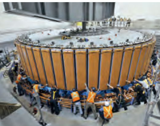
Impressive size – the new rotor is installed in unit 5 of the Revelstoke power plant.
