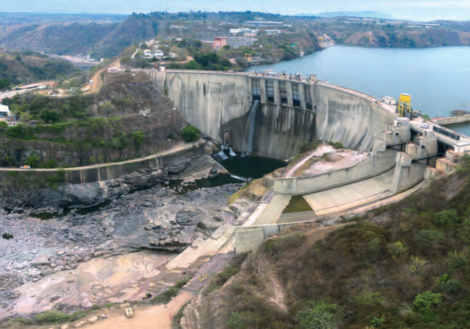
View of the building works at the Cambambe II hydropower plant on the Cuanza River in Angola. The plant is scheduled to start producing electricity with a capacity of 700 megawatts by the end of the year.
