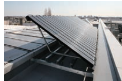
PV solar air panels
