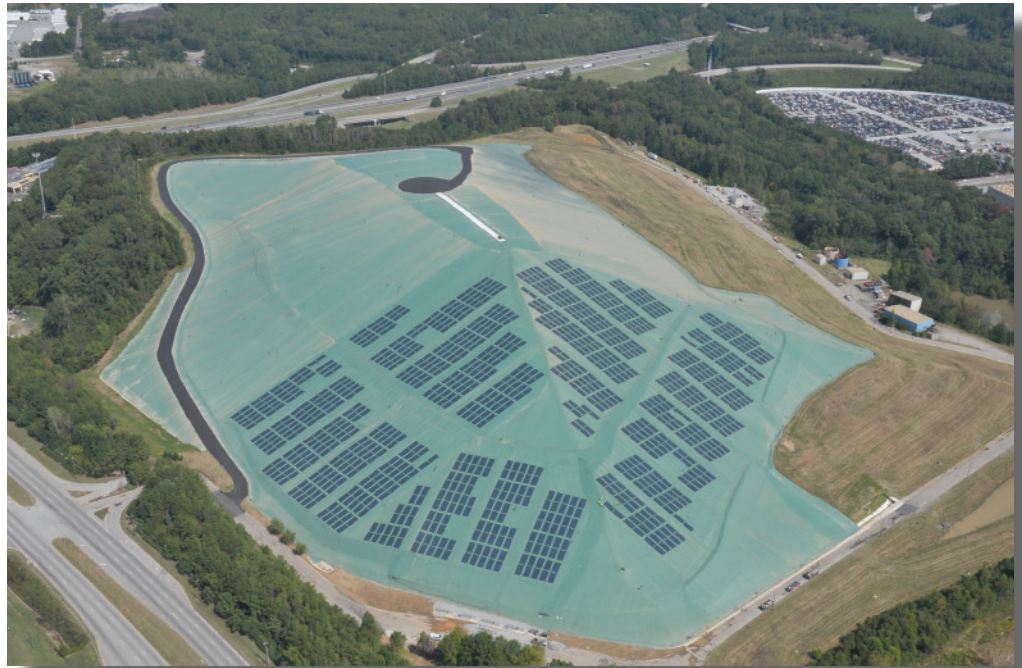
Figure 2: Exposed geomembrane landfill cap with laminated solar photovoltaic panels provides power to serve 224 homes. Photo courtesy of Carlisle Energy Services, Carlisle, PA, www.carlisleenergy.com.
